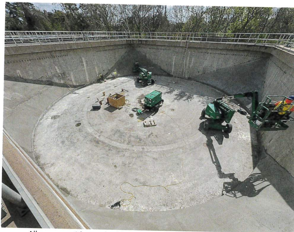
All corners with wrecked forms before clarifier corner inspections.
