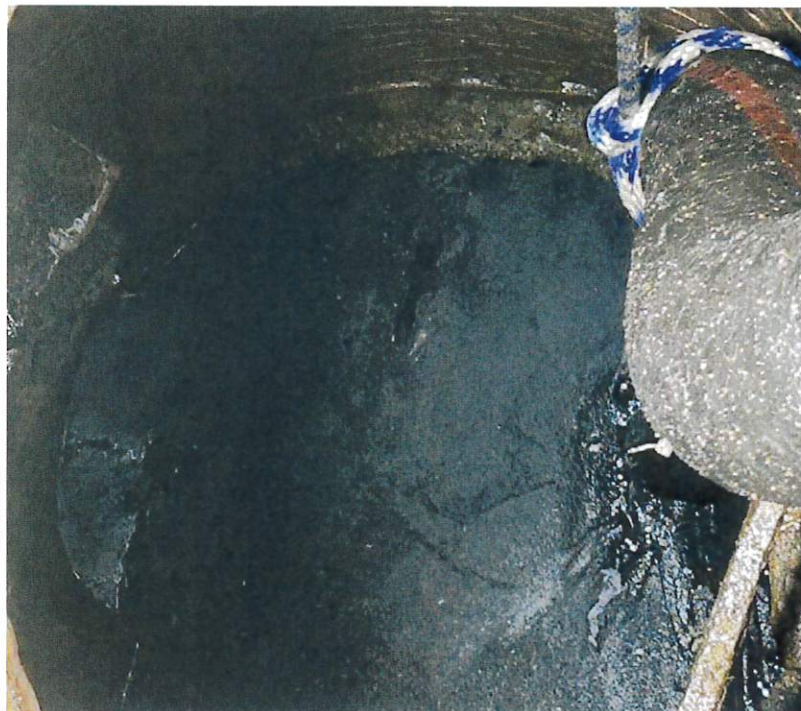
(6/18) – Heavy dirt and debris withing manhole
