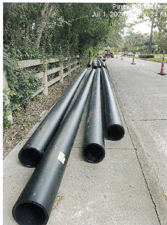
(7/1) – Staging by-pass lines
