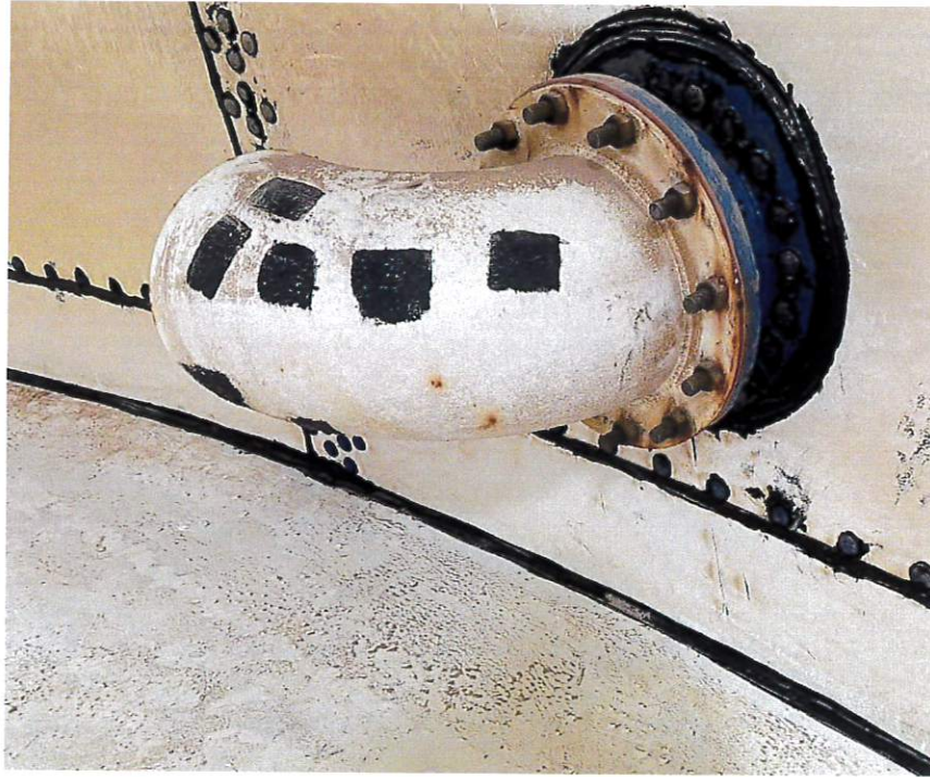
Staining was noted on the well fill line with apparent coating failures.
