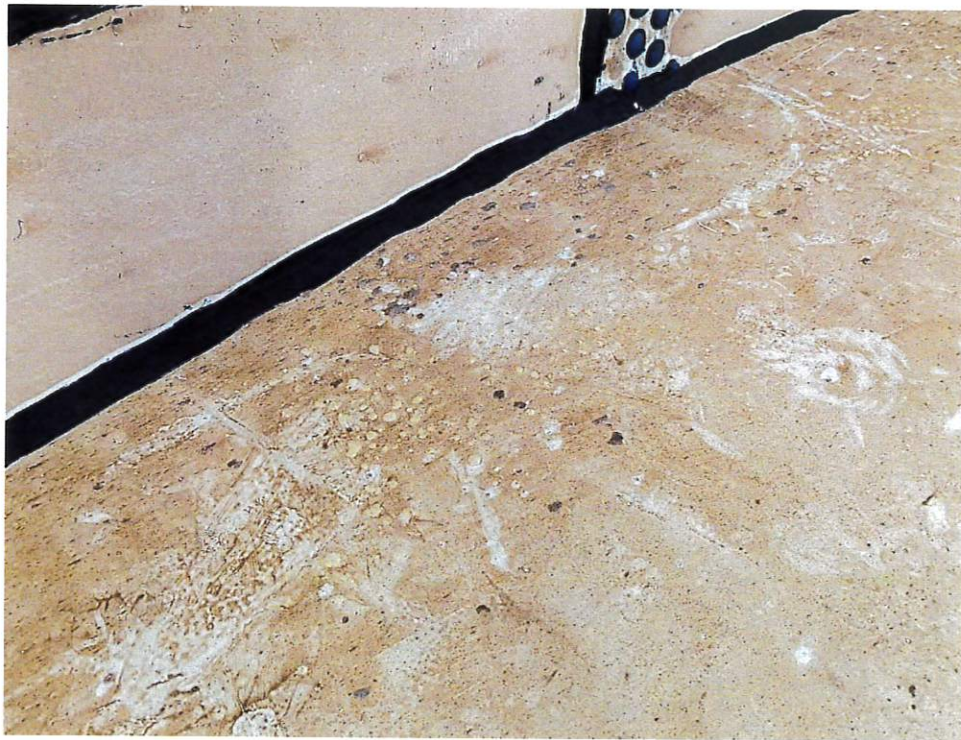
Blisters along perimeter of North GST floor.
