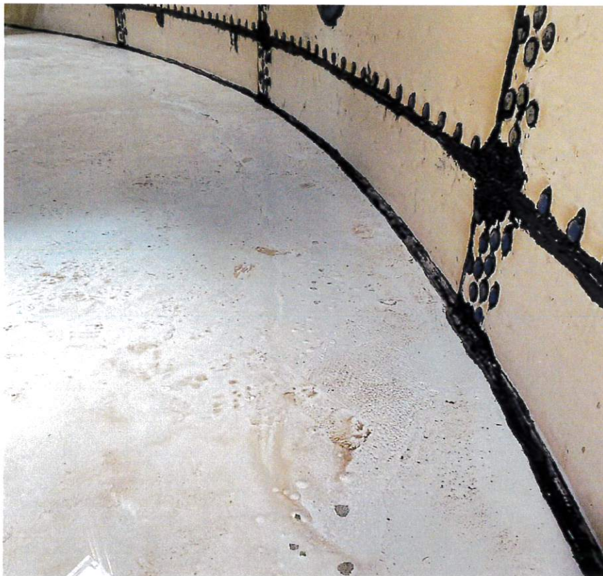
Blisters and additional GST concrete floor failures were noted.
