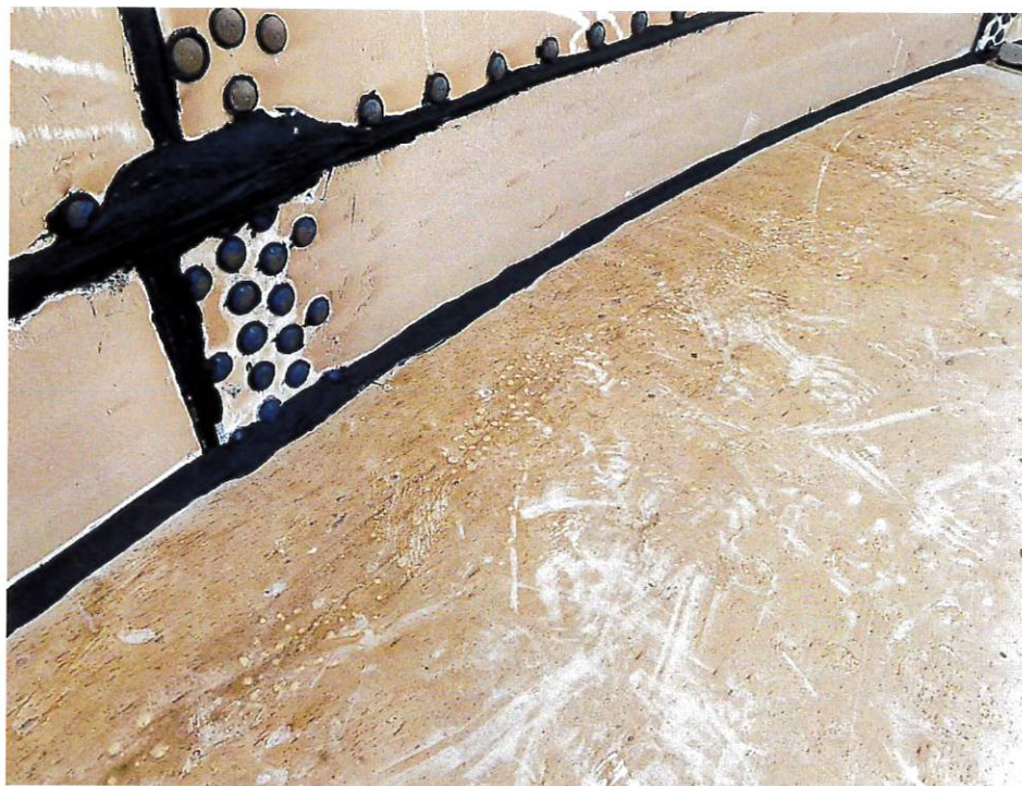
Blisters along perimeter of North GST floor.
