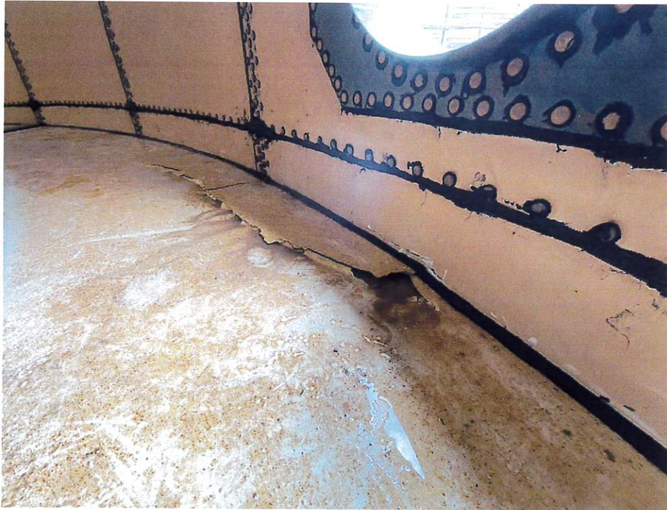
Severe concrete failures and blisters in the coating were noted.
