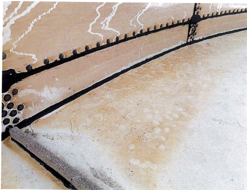
Blisters along perimeter of North GST floor.
