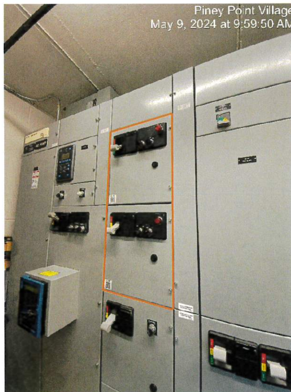
Installed MCC Buckets for proposed Booster Pumps 1 & 2.
