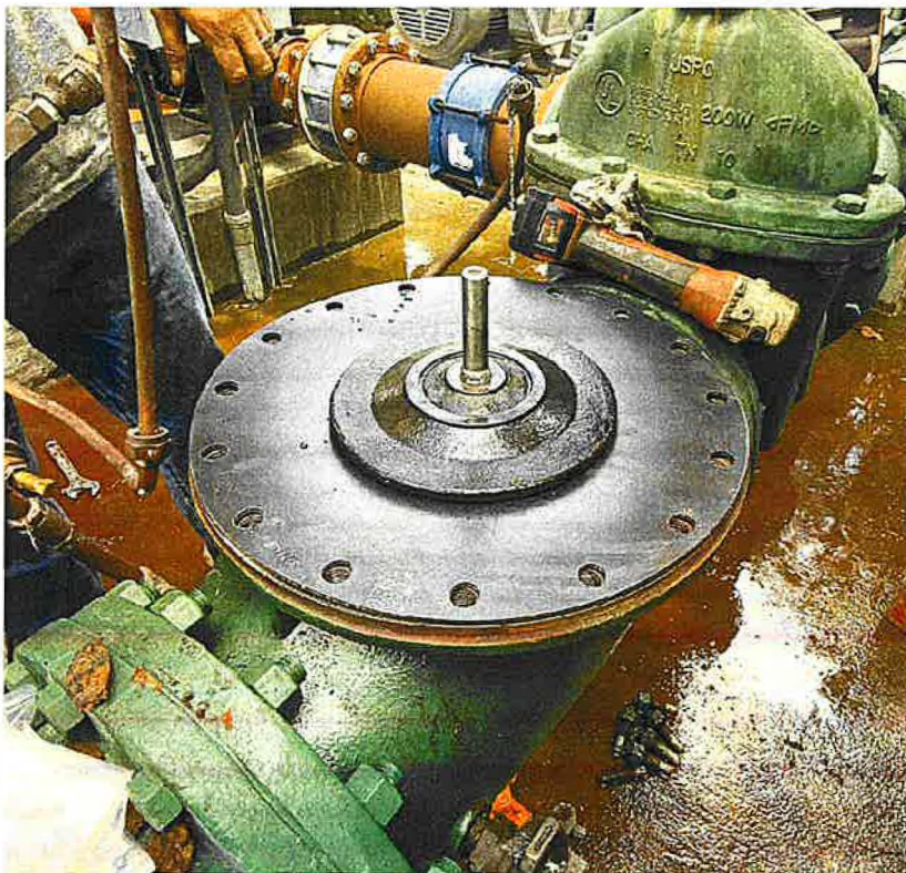
Installed 10" PRV Internal Disc Retainer Diaphragm, as approved via Change Order No. 3.
